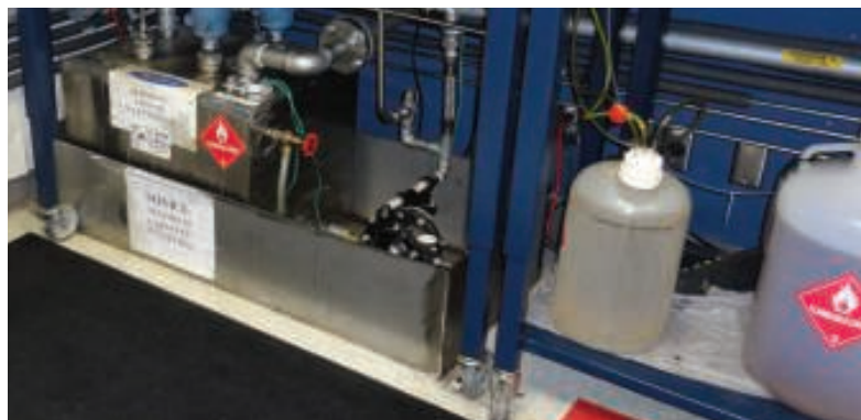
FIGURE 7. The spill containment on the left meets almost all the requirements for effectiveness, although it still requires manual clean up with a rag or absorbent pad. The area on the right, unfortunately lacks sufficient protection
