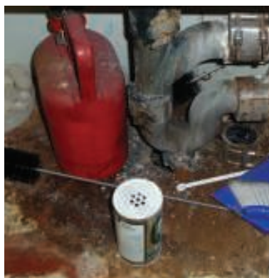
FIGURE 8. Shown here is an example of a spill that can easily leak through the unsealed hole around the drain beside it
