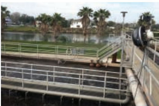
FIGURE 1. Wastewater treatment plants can be sources of odor-causing gases, such as hydrogen sulfide, ammonia, mercaptans and others
