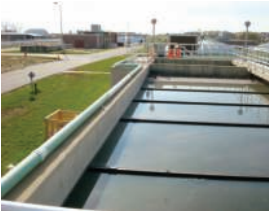
FIGURE 2. Odor-removal methods, such as the vapor-line system shown here, involve treating the air that contains the odor-causing species
