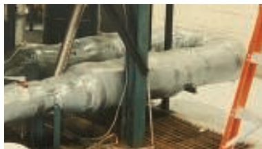
FIGURE 10. Note the modifications extending outside the spill containment
